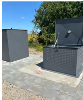
Den nye pumpestation
